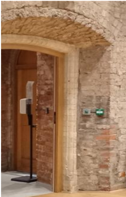
Fig 3. St Peter's Halle doorway, defects observed on the historic fabric during the students' visit. (Maria Yioutani-Iacovides, 2022).
